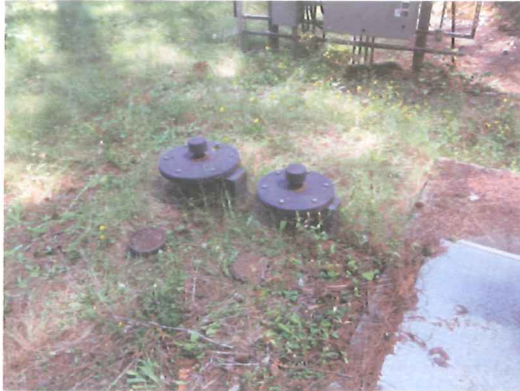
Booster Station Vertical Pitless Pumps
