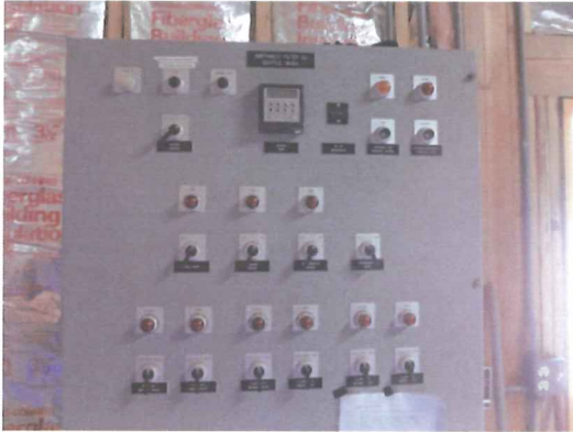
Well #2 Treatment Control Panel
