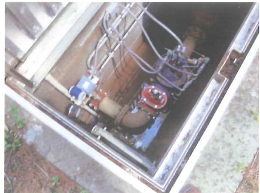
Booster Station Vault
