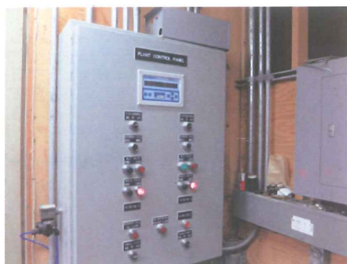
Well #1 Treatment Control Panel
