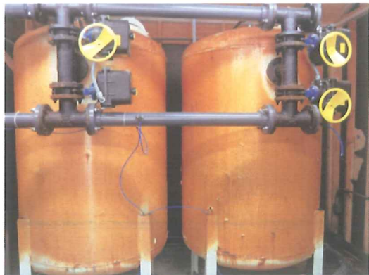
Well #1 Treatment Vessels
