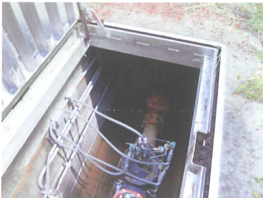
Booster Station Vault
