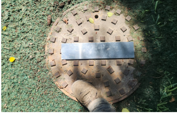
Storm water access, formerly labeled “SEWER”
