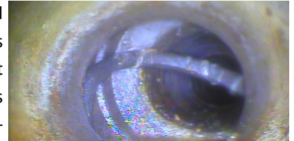
Sewer line break, misplaced gasket a potential to cause blockage
