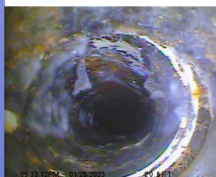
Sewer pipe connection shifted out of place, root infiltration
