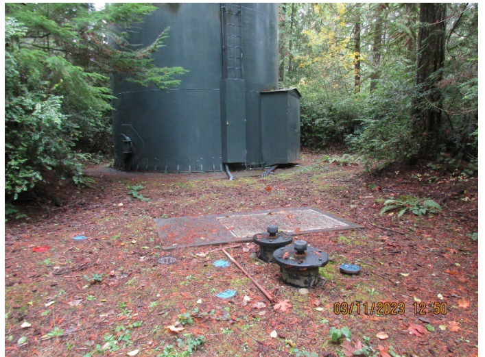
Base of reservoir with off-line "pit" booster station
