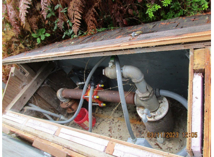
Well 2 well head and enclosure
