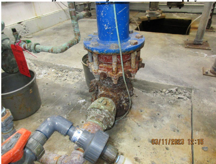
Treated water fitting badly corroded. Will be replaced
