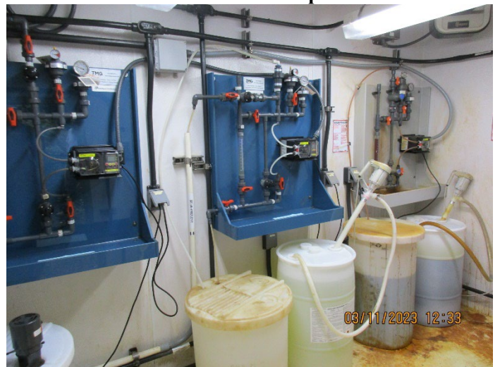
NaOCl, FeCl2, and KMnO4 feed equipment room
