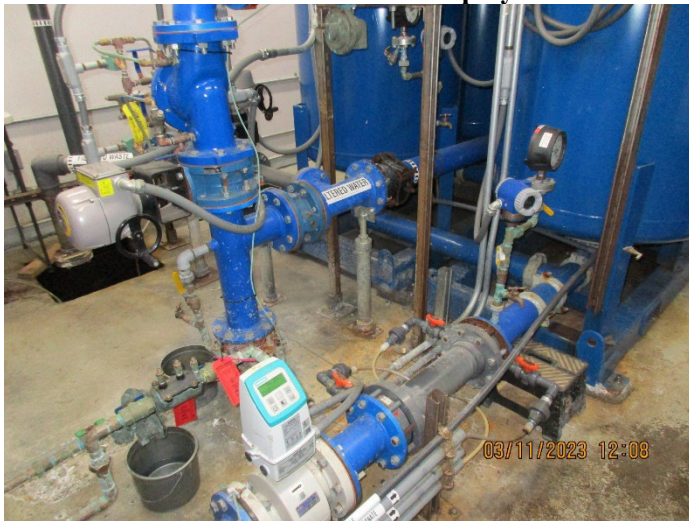
Metering and chem injection of Well 2 supply
