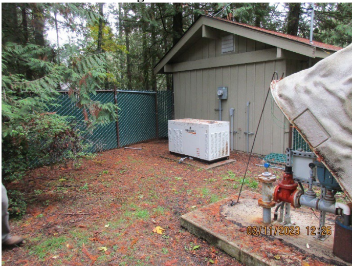
Well 4 and Well 4 WTP generator
