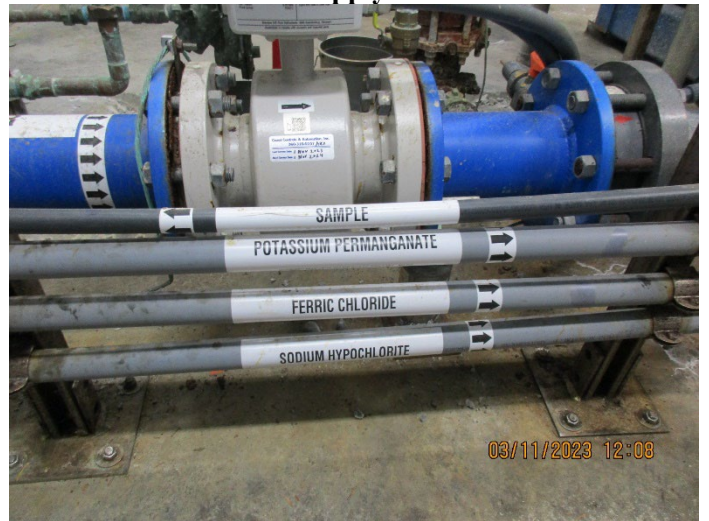
Chemical feed line sleeves and production meter
