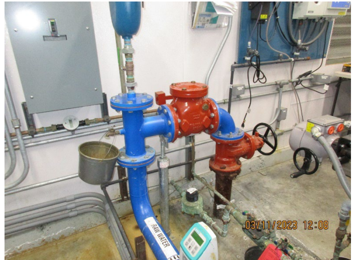
Well 2 supply to WTP
