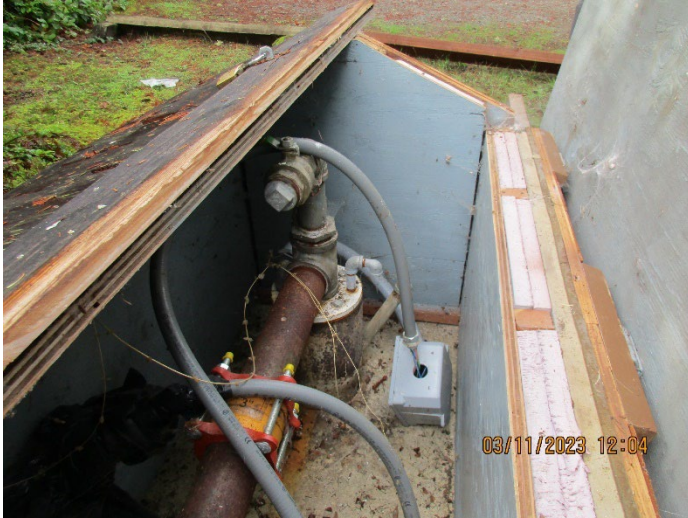
Well 2 well head and enclosure
