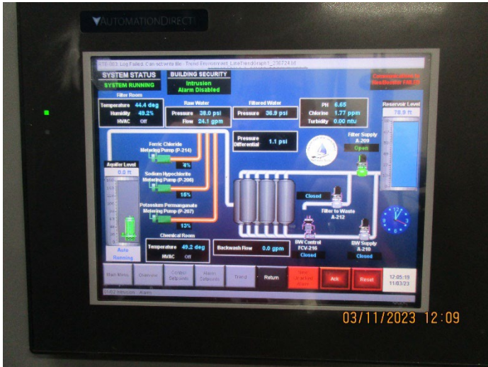
Well #2 WTP PLC display
