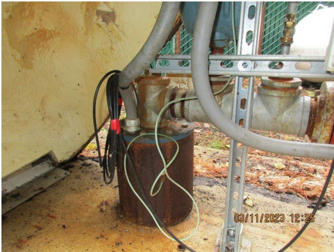
Well 4 well head. Instrument cable (black) entered well casing measures water level
